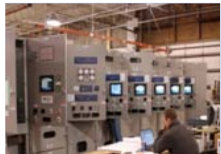
Above: Testing Enercon switchgear technology.
