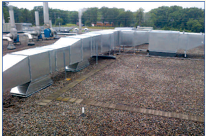
Rooftop Boiler Heat Recovery Unit
