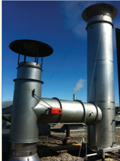
Upgraded Air Makeup Unit
