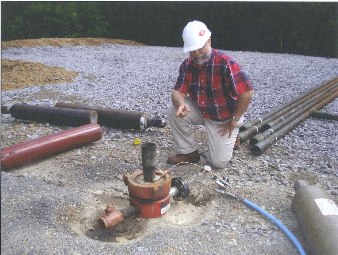
Dr. Jack Pashin, GSA, explaining the pressure gauges and gas sampling lines at the 1-South monitoring well.
