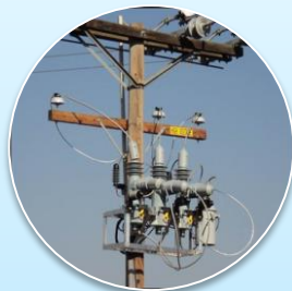
Fault Location, Isolation, and Service Restoration
