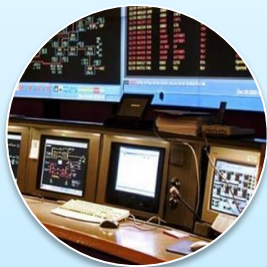
Advanced Distribution Management System (ADMS)
